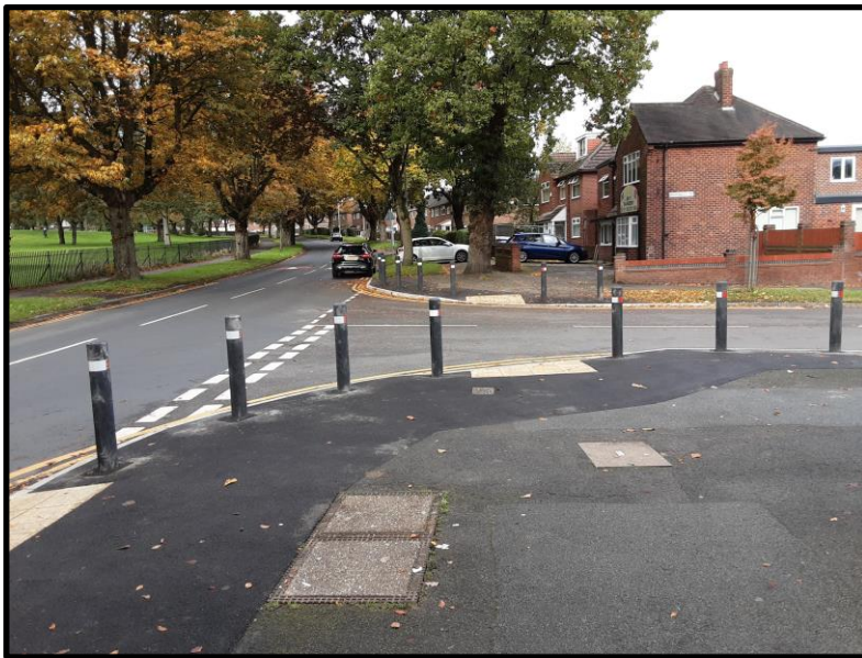
Firbank Road/Highdales Road, Baguley - Reconfigured junction/bollards/drop kerbs/tactile pavings/road markings/traffic signs/No Waiting at any time restrictions
